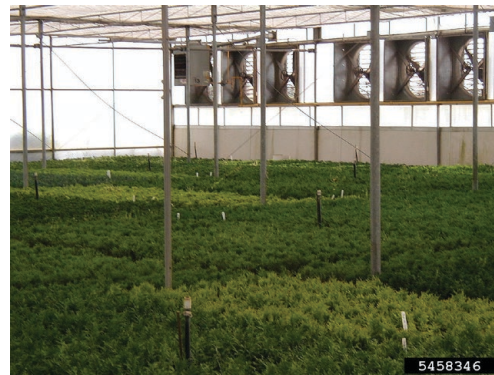
Figure 2. Exhaust fans placed in the endwall of a greenhouse pull warm, moist air out of the greenhouse. Rachel McCarthy, Cornell University, Bugwood.org.
